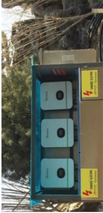
15kw three-phase system
